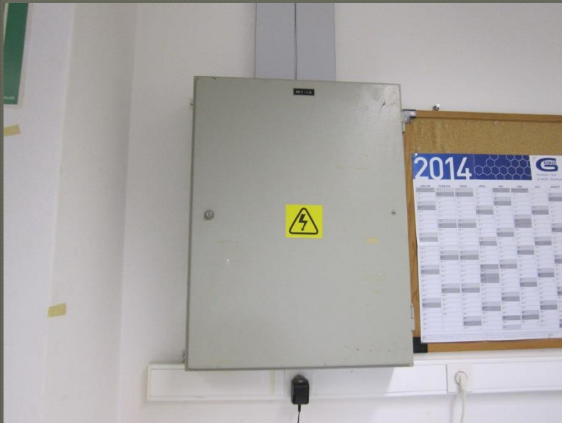
Electrical panel – warning sign Easy to access
