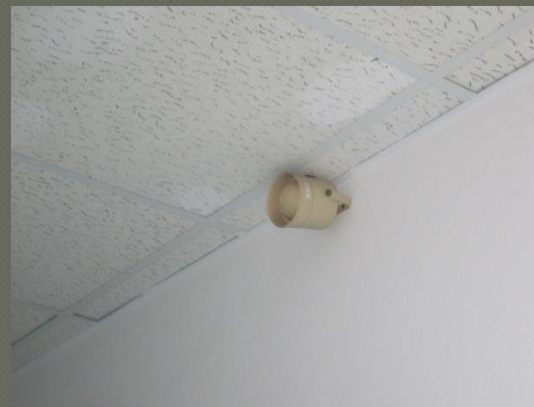
Fire alarm signal
