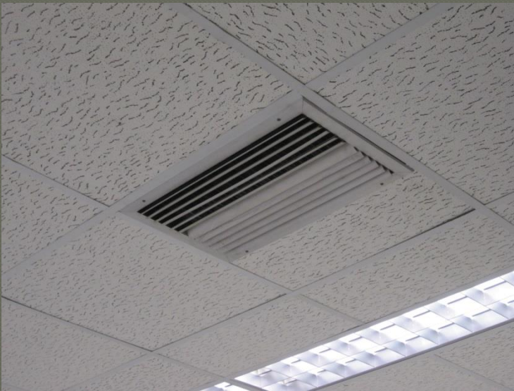
Air inlet in ceiling
